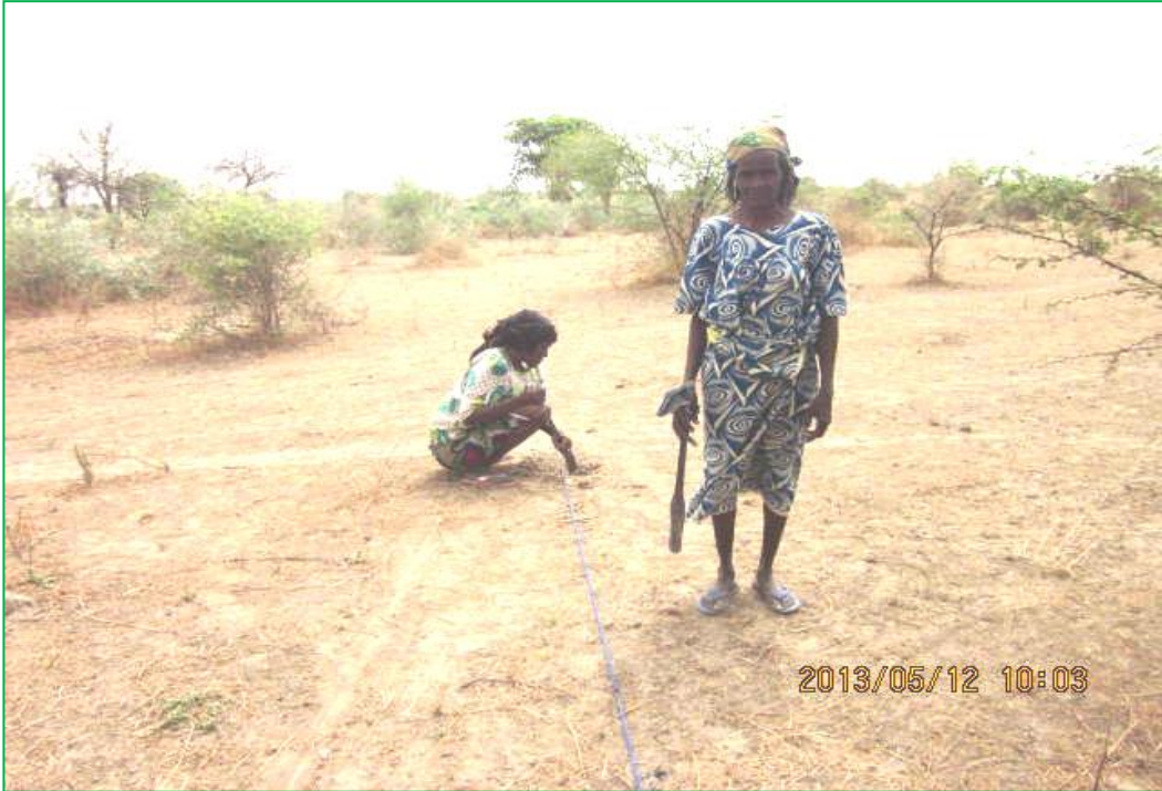
The work of clearing and staking site: the village women were present and actively participated in the project work.
